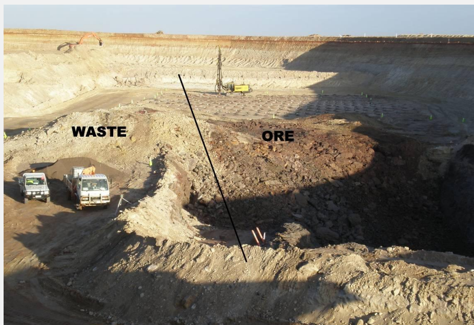
Figure 4: First blast (looking west), showing nominal ore / waste boundary. The ore dips to the left of photo
